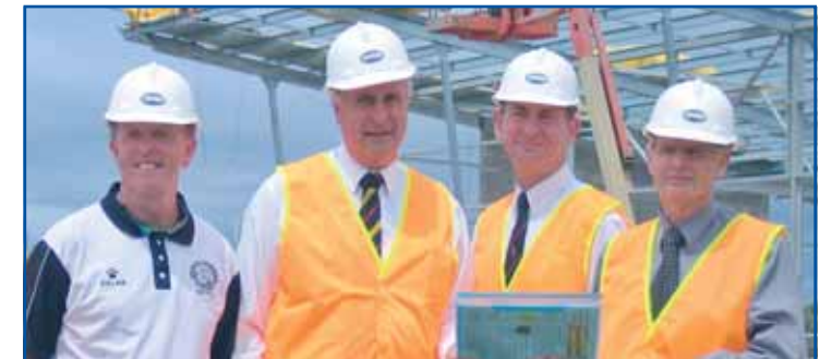
John Fitzmaurice, Mr Randall, PACC Executive Officer Patrick Gallagher and City of Mandurah Director of Community and Economic Development Ian Hill see the sporting complex take shape
